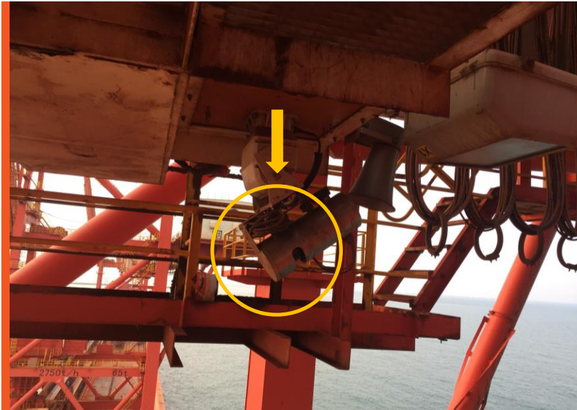
Quanergy M-series 3D LiDAR sensor mounted on a pitch control equipment with a protective cover
